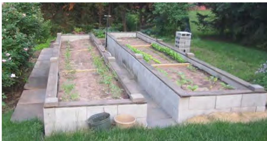
Due to the grade, the third course is under ground in the front while above ground in the back of the raised beds.
