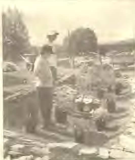
Susan Munger and Mike Dietz checking on the placement of plants to be installed in the rain garden
